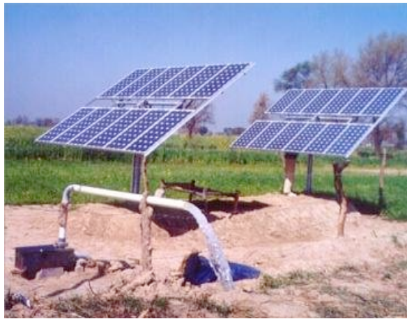
Solar water pumping installation in Chongwe
